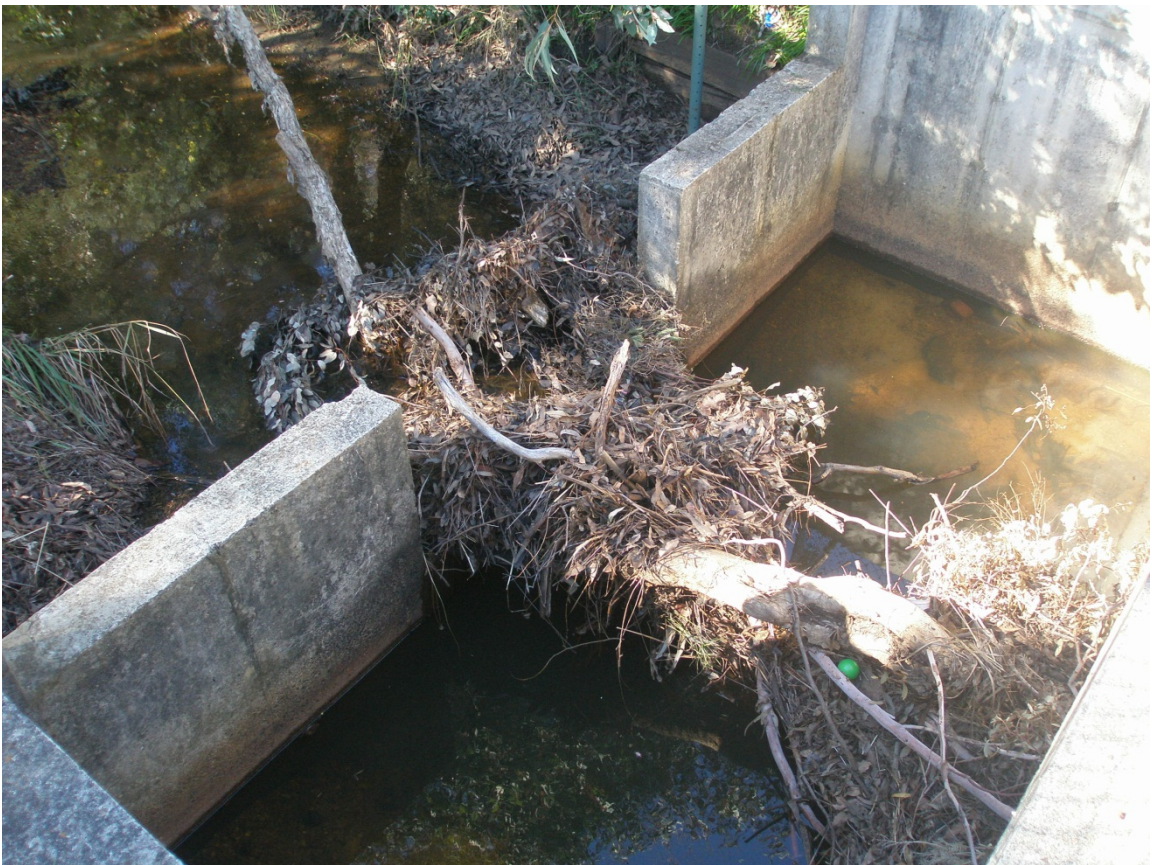
Photograph 11 and 12: Debris collected on the weir and potentially affecting stage discharge relationships at Site M1 in June 2009
