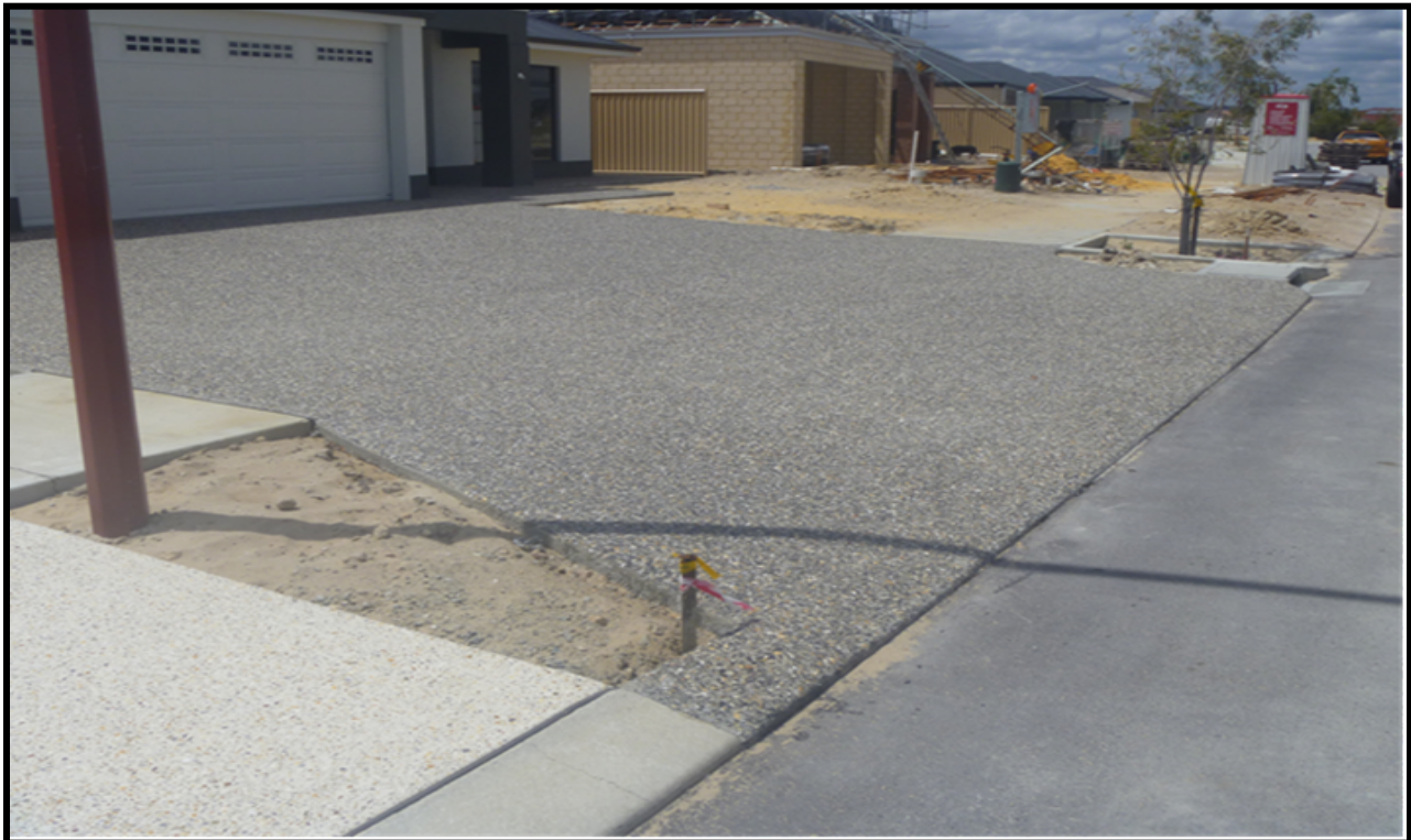
Figure 6 - Crossing constructed through path, too wide, too close to side entry pit and incorrect kerb replacement- Non-compliant
