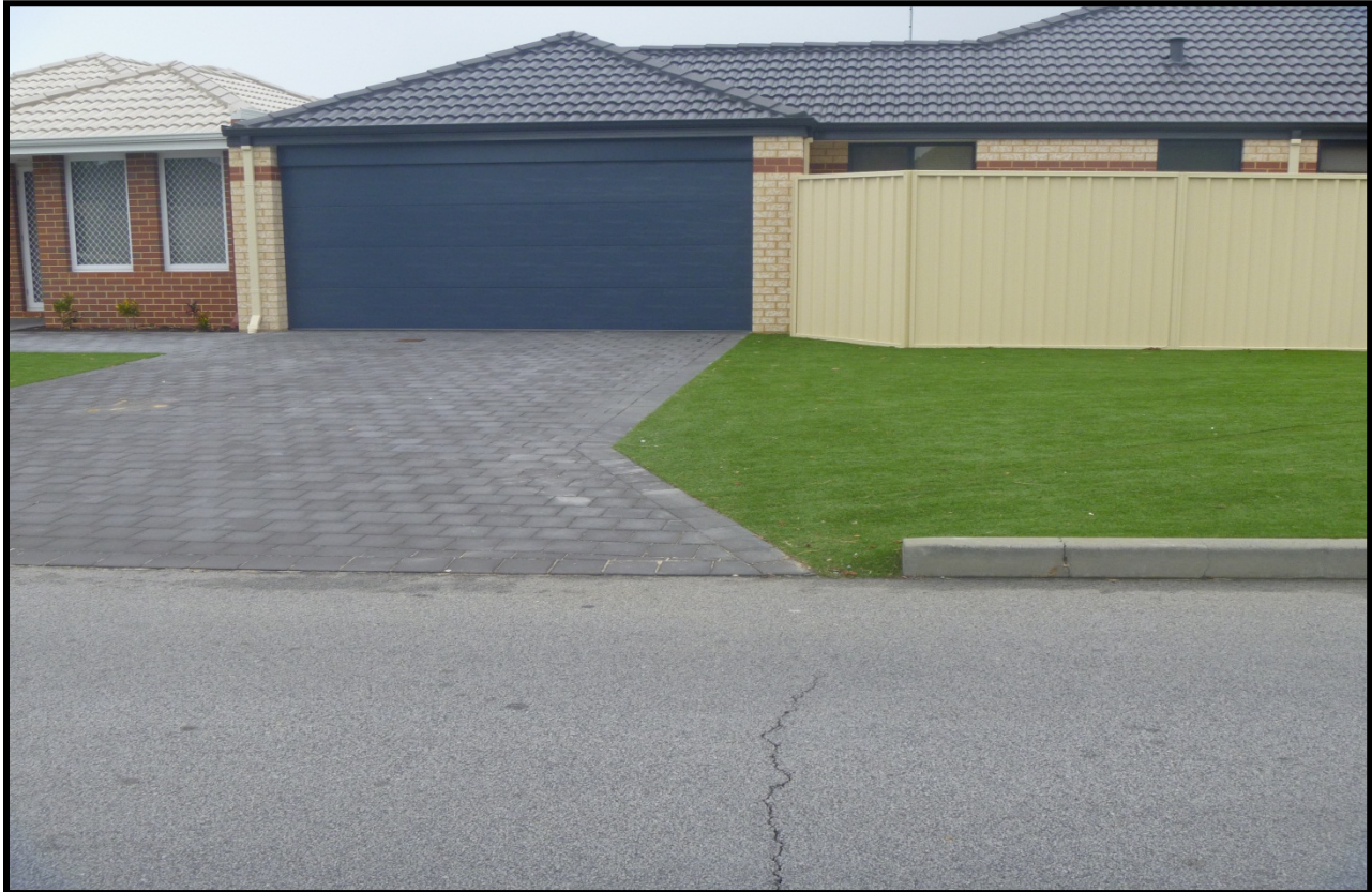
Figure 5 - No kerb - Non- Compliant
